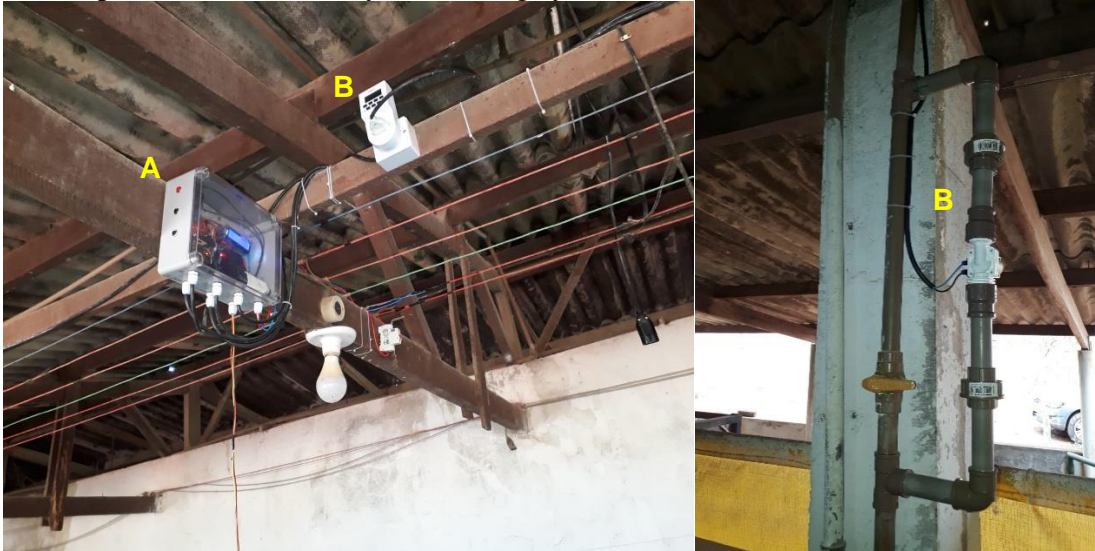
Figure 1. Temperature and humidity monitoring system.
