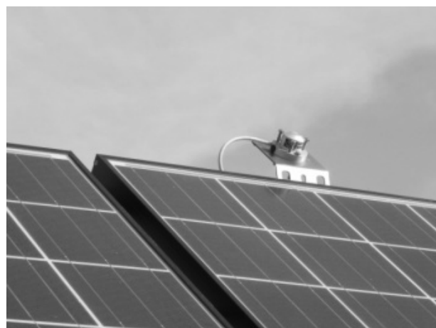
Figure 8 - Pyranometer installed on the same plane of the Photovoltaic generator.
